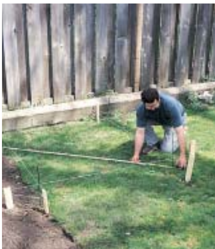
A. Lay out the location of the arbor posts, then measure the diagonals to check for square.
