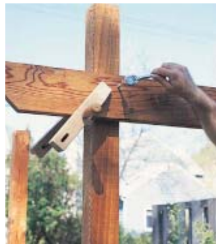
C. Level and clamp the tie beam against the posts, then secure it with lag screws.
