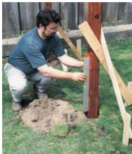
B. Brace the posts into place, then use a level to make sure they are plumb.
