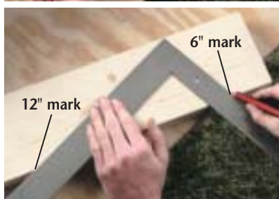
A. Position the framing square at the 6" and 12" marks to draw the top and bottom plumb-cut lines.
