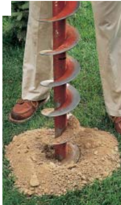
B. Dig post holes 6" deeper than specified by local building code. Pour 6" of gravel into each hole to improve drainage.
