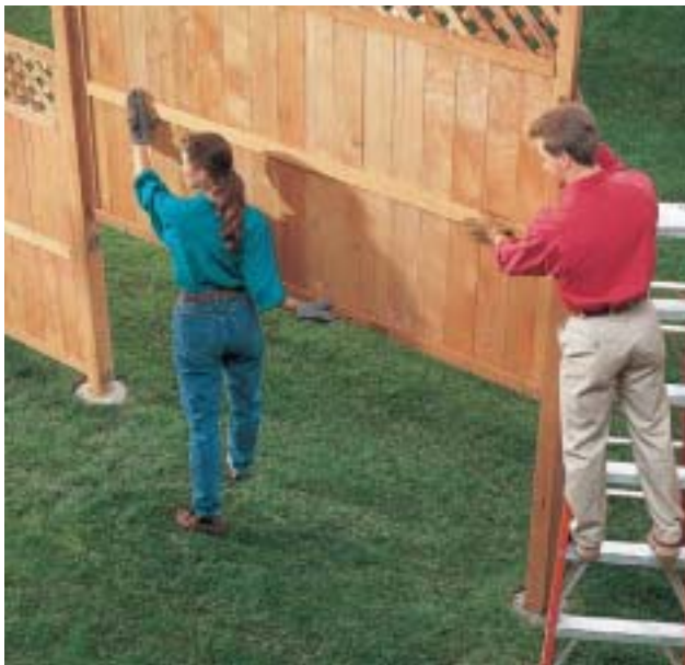
C. Slide the fence panels into the brackets from above, until they rest on the bottom flanges of the lowest brackets.
