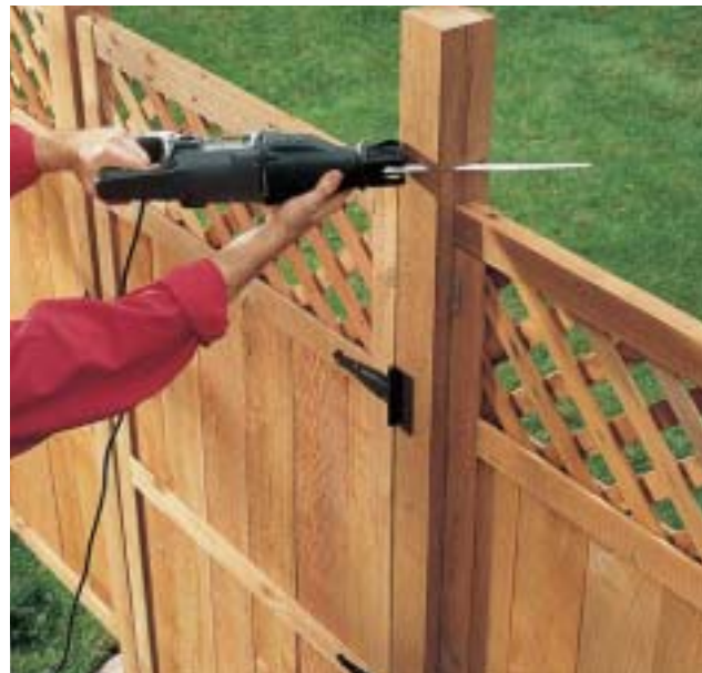
E. Trim the post tops to size, using a reciprocating saw. Cover each post top with a decorative post cap, or trim it to a point to help shed water. Paint or coat the fence with sealer.
