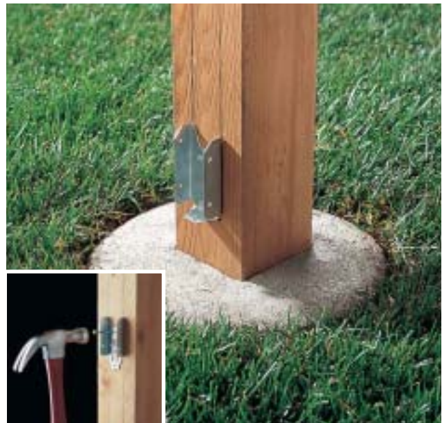
B. Align the bottom of the first bracket 2" above ground level. Evenly space two more brackets inside the outline, attaching each bracket with 4d galvanized nail (inset).
